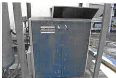
Compresor original nefunctional
